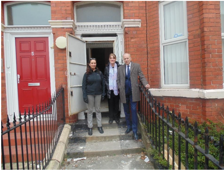
Committee members Liz Smith, Cynthia Pugh and John Fairhurst outside 7 Kelvin Grove as work commences on the first refurbishment
